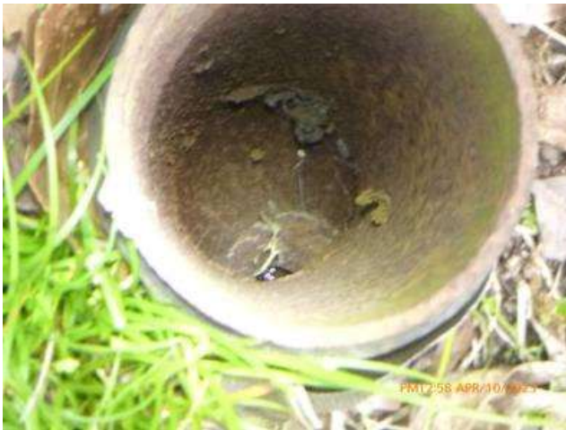
An open sewer pipe was observed in the backyard. These sewer access cleanouts are normally capped.
