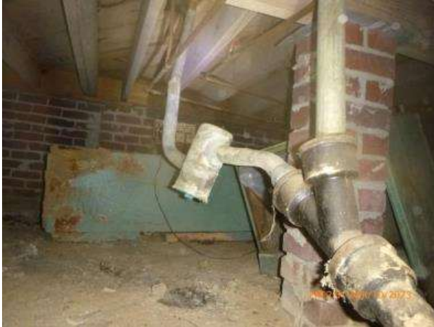
An obsolete drum trap was observed. This device has a history of failing to perform properly.
